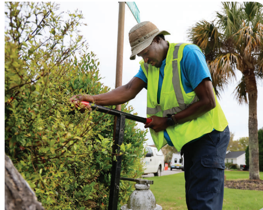
Hydrant Maintenance Operator John Bennett and his crew team members have to open fire hydrants to flush them.
